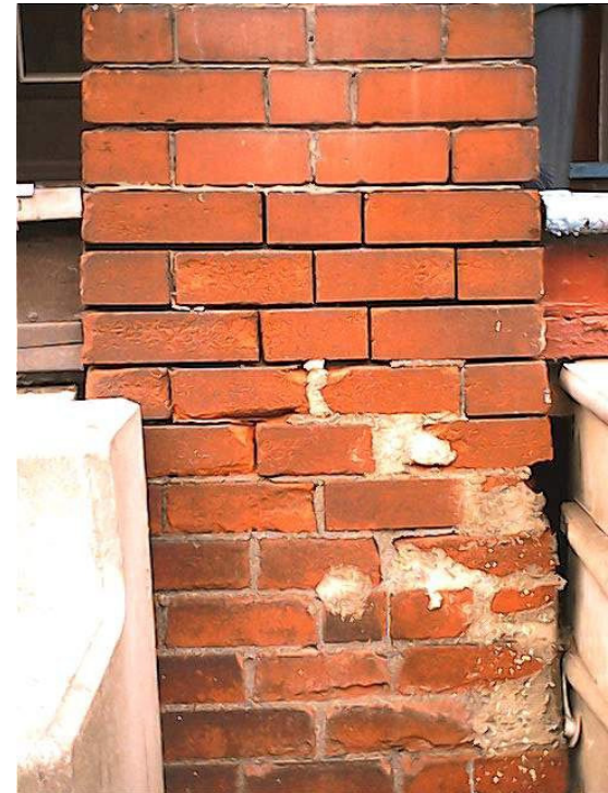
Progressive deterioration: Rainwater splashing on the porch and steps eroded the mortar. That let increasing amounts of water into the bricks and mortar below, and they are spalling and washing away, letting in even more moisture.
