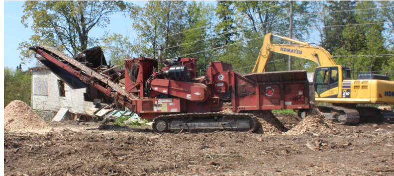
Demolition of an unsalvageable former cottage building near Duffins Creek in Ajax
